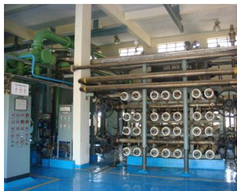
1.8MLD SWRO Desalination Plant at NDDP, Kalpakkam
