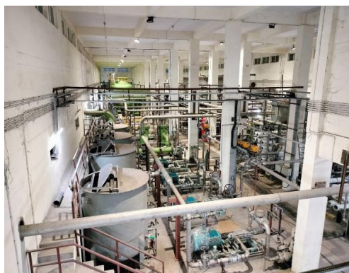
4.5MLD SWRO Desalination Plant at OSCOM, Orissa
